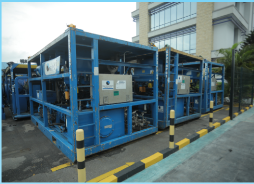
180K Zone 2 Nitrogen Converter Pumps delivering upto 180,000 scf/hr
