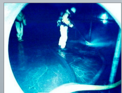
A high-pressure jetting operation in a storage tank using retro jetting gun
