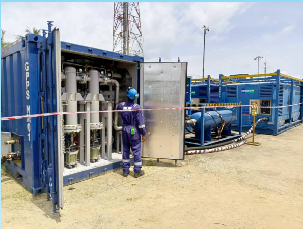
Overview of GPPS Nitrogen generation project in a clients facility membrane
