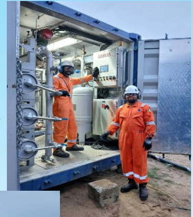
Nitrogen membrane with the operators on site in a nitrogen supply project
