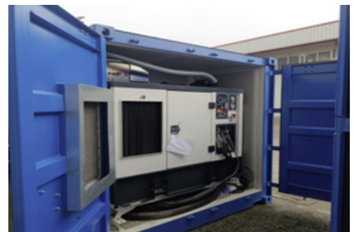
Atex Zone 1 10ft marine container with ergonomic controls cabin installation
