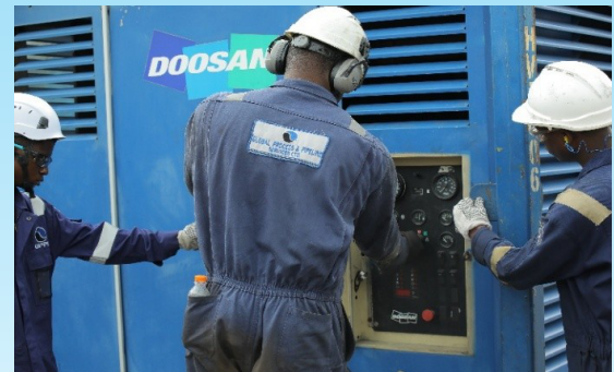
Highly trained and competent Operators supplying compressor air in a clients facility
