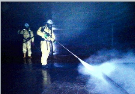
Personnel in tank cleaning operation during a finishing touch after sludge/slurry evacuation
